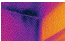
Termite Nest located via thermal imagery
